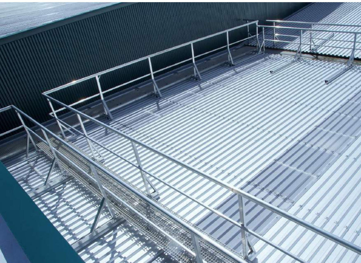
Aluminium Walk-way Mounted Handrails at Bunnings Hamilton.
