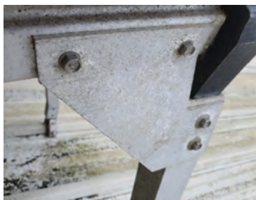
FIGURE 3 PRODUCT INSTALLED IN A HIGHLY CORROSIVE DAIRY PLANT ENVIRONMENT 16 YEARS -NO CLEANING
